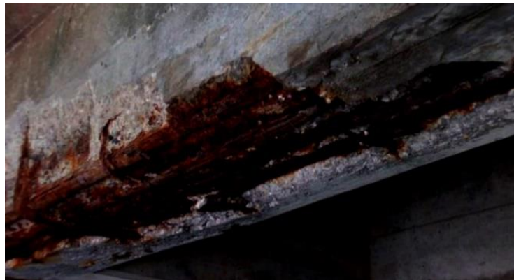
Fig. 1. Reinforcement corrosion seriously undermines the performance of an RC structure.
