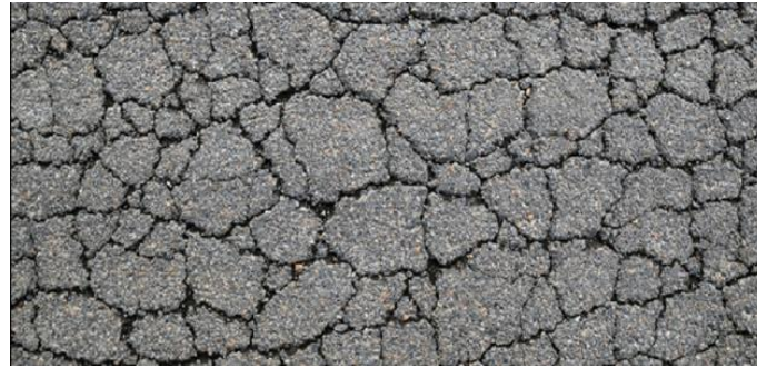
Fig. 7. Mosaic cracks or lizard skin.
