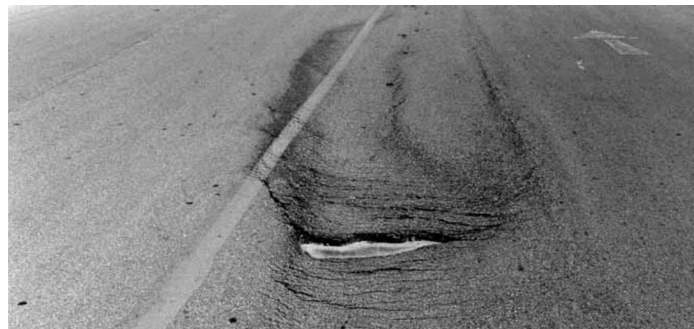
Fig. 6. Cracks resulting from the sliding of the asphalt layer on the underlying layer.
