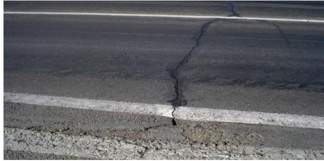
Fig. 4. Longitudinal and transverse cracks.
