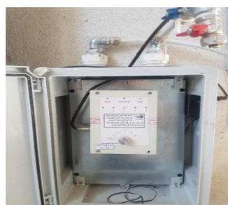
Fig. 7. Magnetized water generation device.
